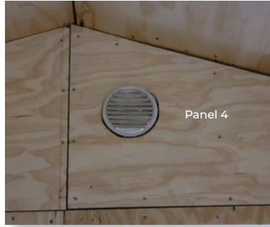
Photo: Louvered Vent on Wall #2
